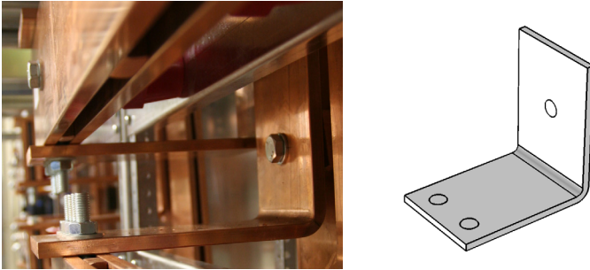
Figure 1: Photo of a busbar installation, and the geometry of the busbar used in this example.
