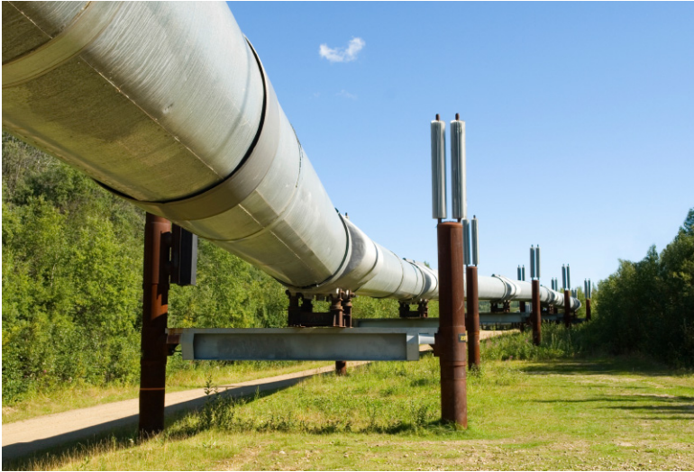
Figure 1: A section of pipeline transporting crude oil.
